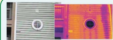
The thermogram of the apartment building shows the path of a serious leak, completely hidden within the wall, from a washing machine on the third floor
